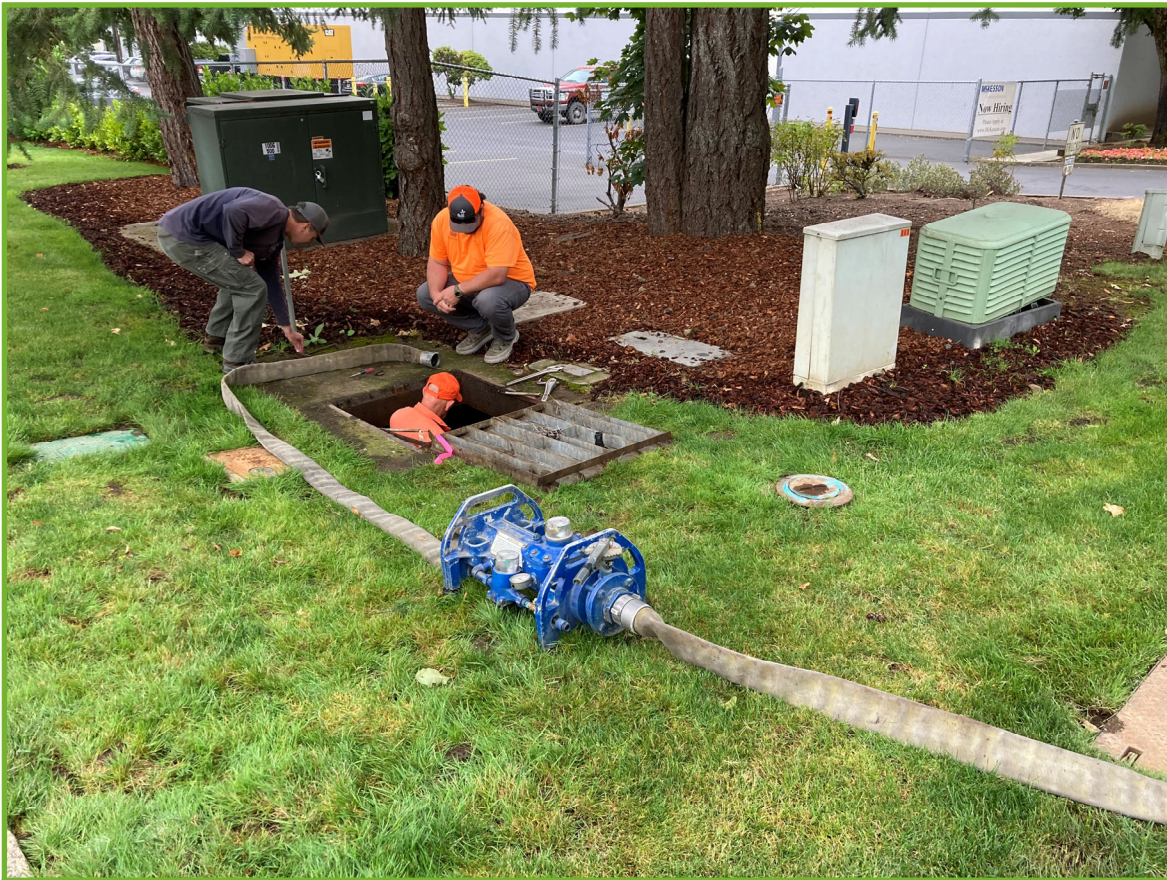
Testing a large meter on commercial property
