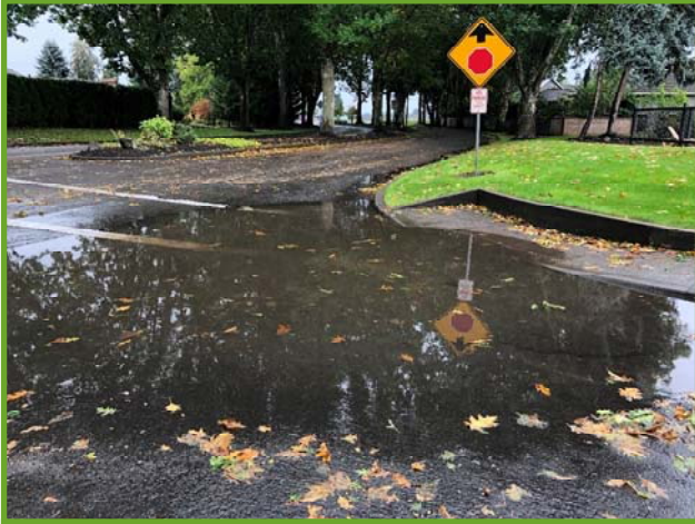
Standing water at crosswalk
