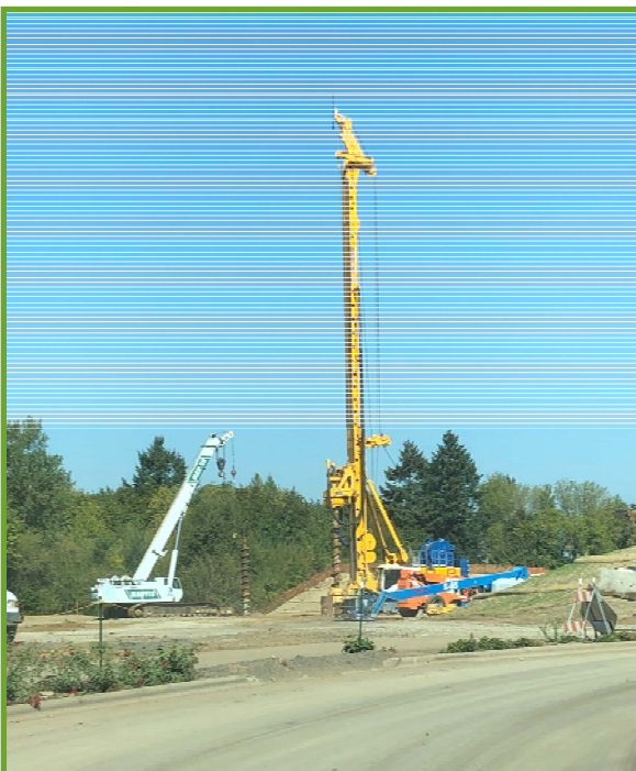
Drill rig and crane on upper site for trenchless crossing under Arrowhead Creek
