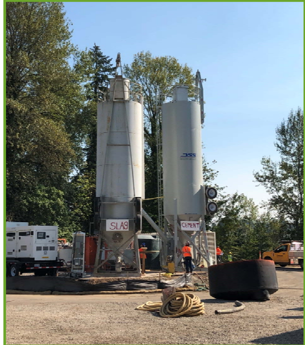
Mixing plant to create slurry for the deep soil mixing along the Willamette River bank
