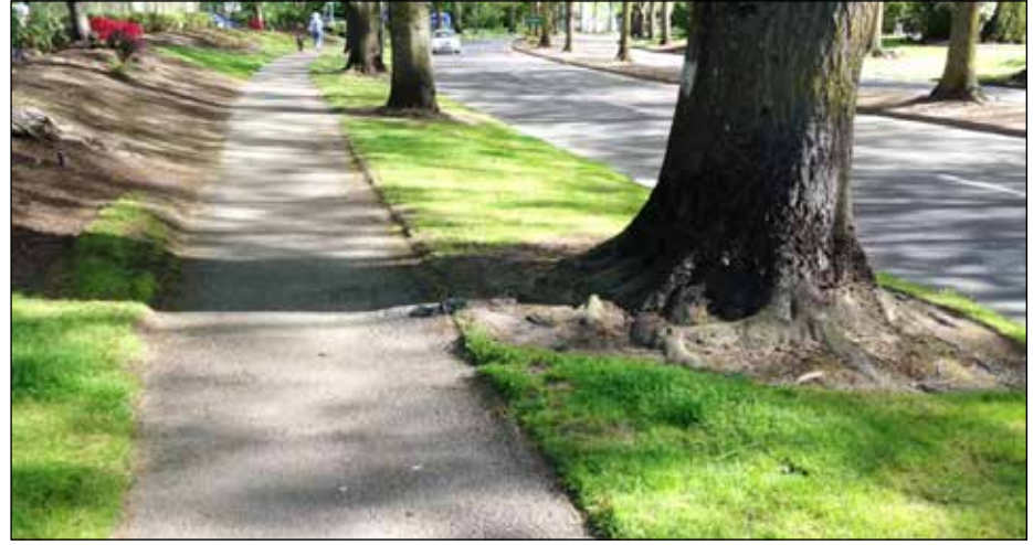
Pedestrian pathways serving Charbonneau on French Prairie Road were largely built in the 1970s, and lack modern conveniences for cyclist and pedestrian safety.
