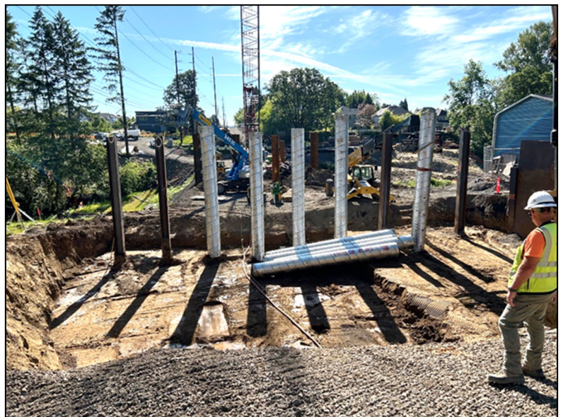
Construction of the west bridge approach is underway with excavation complete, piles installed, and pile sleeves going over the piles.
