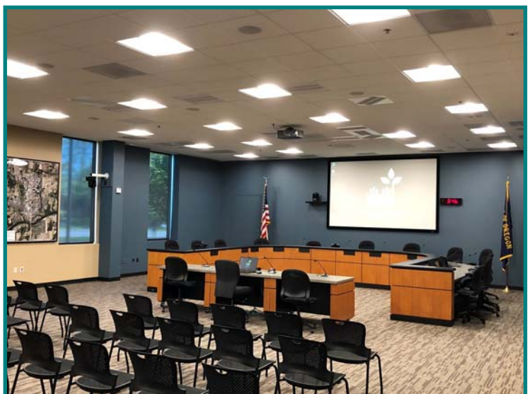
After (LED lights) - Council Chambers
