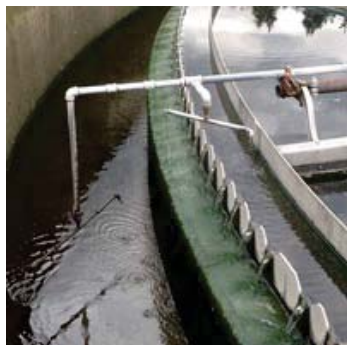
Secondary clarifier 1 weir washer
