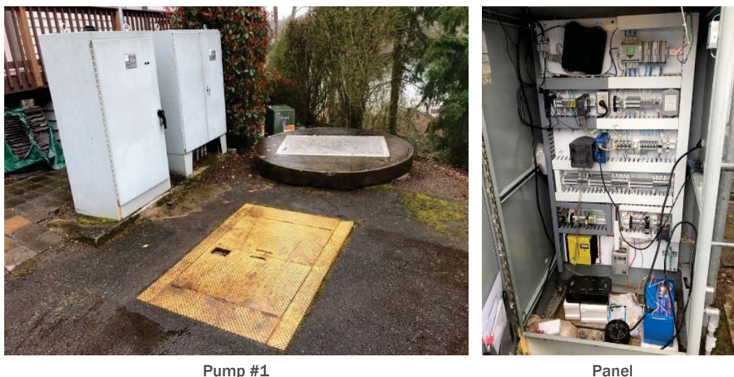
Figure 4-7. Rivergreen Lift Station
