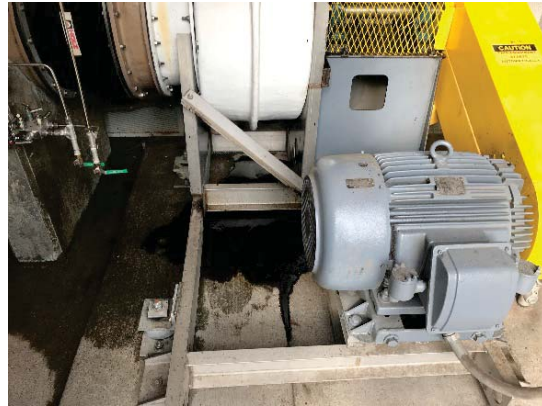
Oily residue at odor control fan
