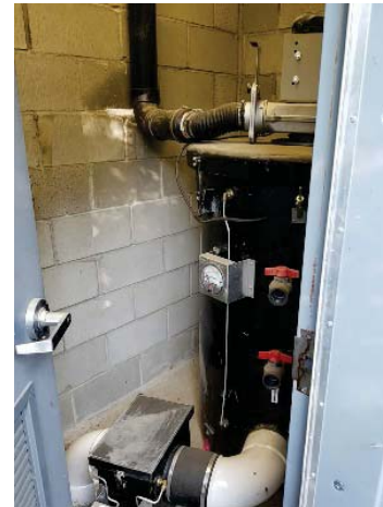
Odor control unit
