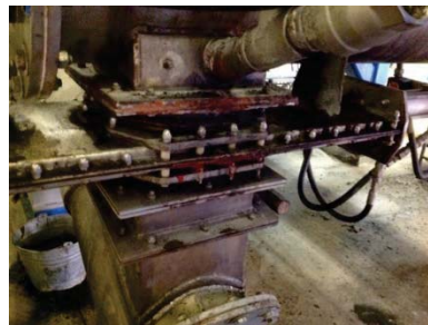
Dryer discharge conveyor
