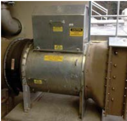
Aeration Basin Emergency Bypass Fan
