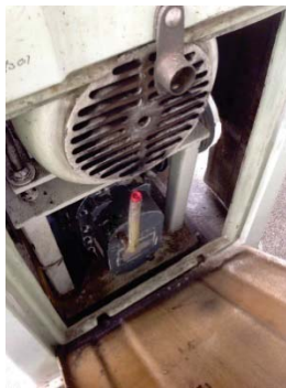
Biosolids storage blower 2
