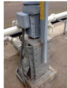
Centrifuge feed pump 2
