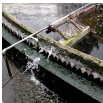
Secondary clarifier 2 weir washer
