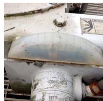
Secondary clarifier 2 torque meter
