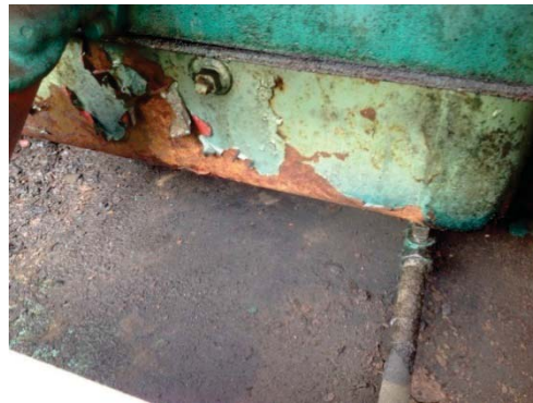
Onan portable gas generator
