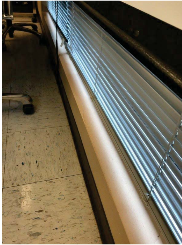
Windows under screen seem to be leaking
