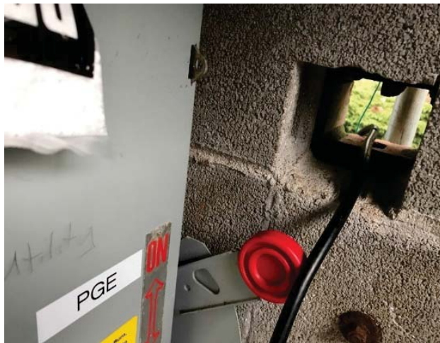
Antenna wire and power disconnect
