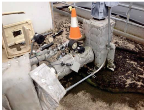
Centrifuge feed pump 1
