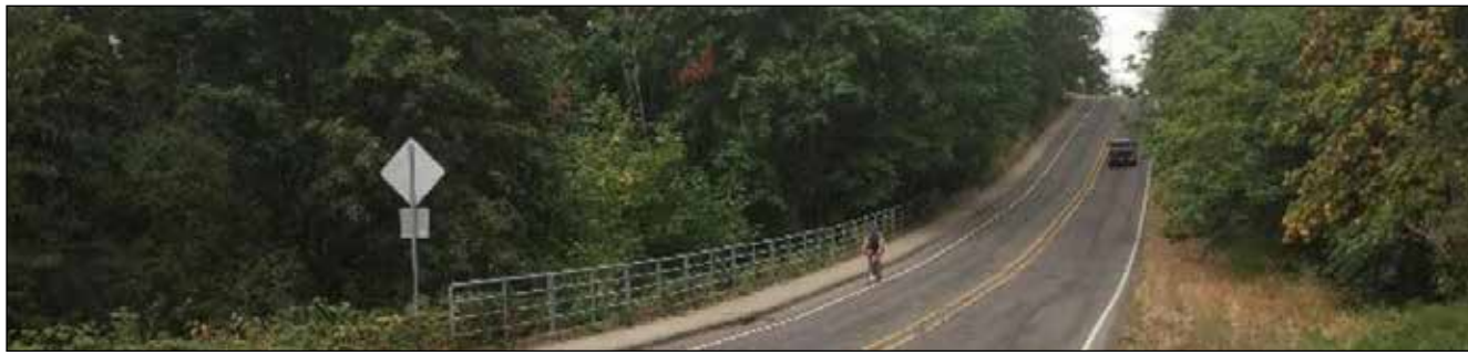
The portion of Boeckman Rd. that includes the "Boeckman Dip" is undergoing several improvements, including a bridge to flatten the curve and provide passage for wildlife. The upgraded road includes dedicated bike and pedestrian lanes.
