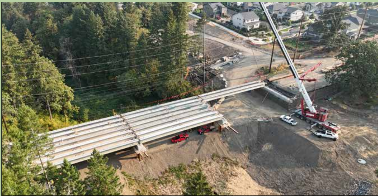
A drone's-eye view of construction at the Boeckman Dip Bridge shows bridge girders being installed in early September. The major project to upgrade the City's road infrastructure is scheduled to be completed this spring.
