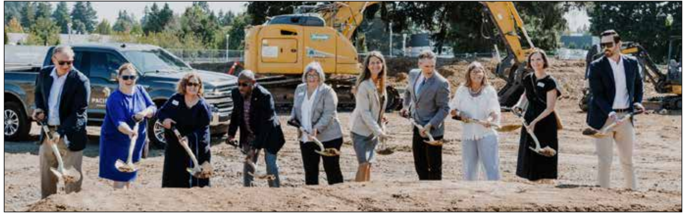
Celebrating the start of construction at Vuela were (from left) Palindrome Vice President, Development, Robert Gibson, Metro Councilor Christine Lewis; Wilsonville City Councilor Caroline Berry; Oregon State Senator Aaron Woods; Wilsonville Mayor Julie Fitzgerald; Oregon State Representative Courtney Neron; Palindrome President Chad Rennaker; Clackamas County Commissioner Martha Schrader; Wilsonville City Council President Kristin Akervall, and Pacificap Construction Director of Construction Ryan Whitt.
