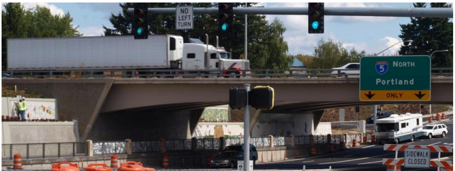
Student-produced artistic tiles being installed at the I-5/Wilsonville Road interchange underpass area, August 2012.
